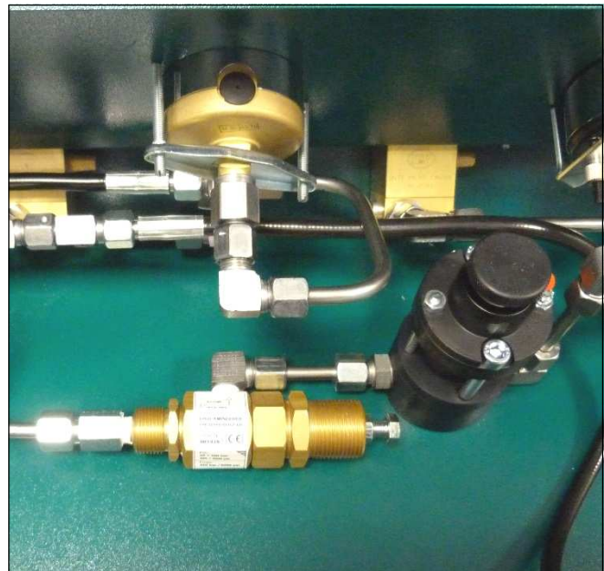
Pressure reducer (left) & safety valve (right)
