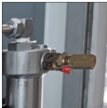
Safety valve 2nd stage
