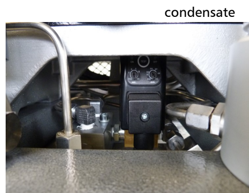
Fig. 2—Timer below the compressor block
