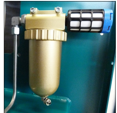
Oil / water separators final stage
