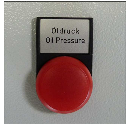
Oil Pressure Monitoring
