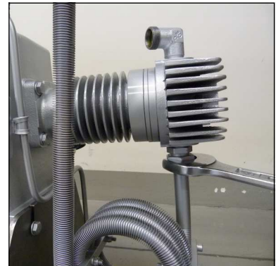
Fig. 4 - Loosen pipe connections
