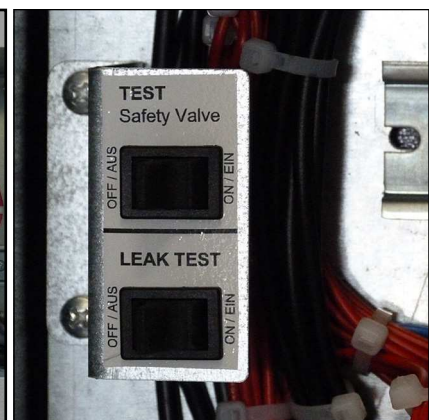
Safety valve test switch (up)
