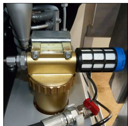
Oil / water separators final stage
