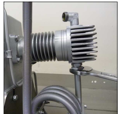
Fig. 3 - Loosen pipe connections
