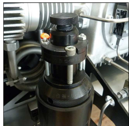
Fig. - Safety valve 3rd stage
