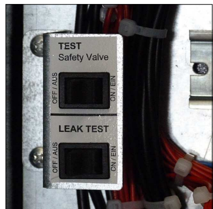
Safety valve test switch (up)
