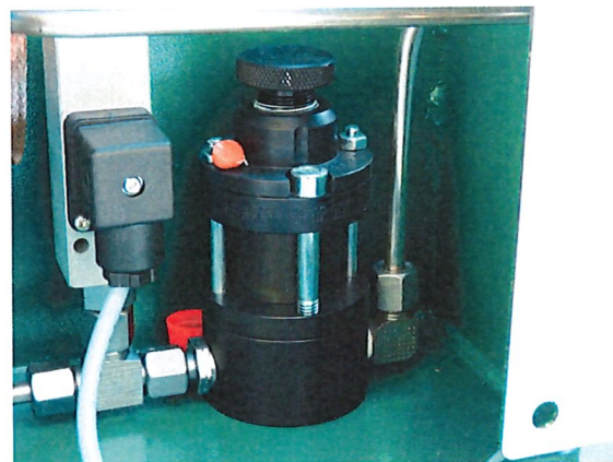
Safety valve final pressure
