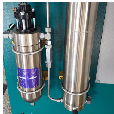
Fig. 3 - Loose pipe connections and nuts
