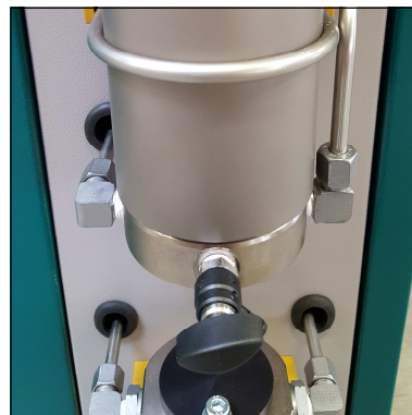
Fig. 3 - Loose pipe connections and nuts
